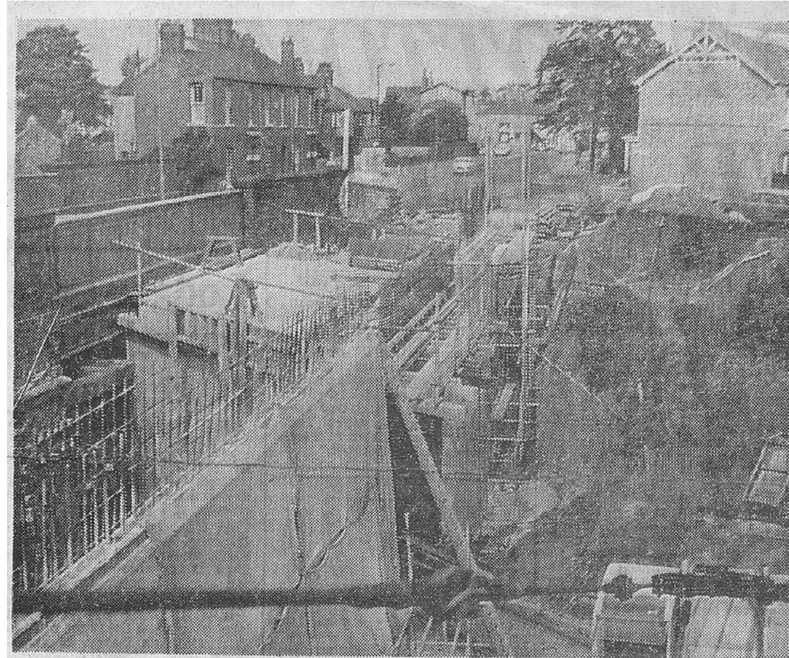
Work on Layerthorpe Bridge, York, has progressed enough to show a new concrete span, which will add to the width of the present road.
